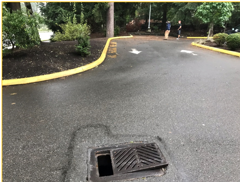
Photo 5C – Looking West – Flows enter the catch basin and is conveyed west into a manhole located in the planter area of parcel 9265030055.
