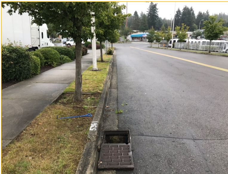
Photo 4A – Looking East – Flows are conveyed east along the north side of S 332 nd Street in a series of catch basins towards Pacific Highway S.
