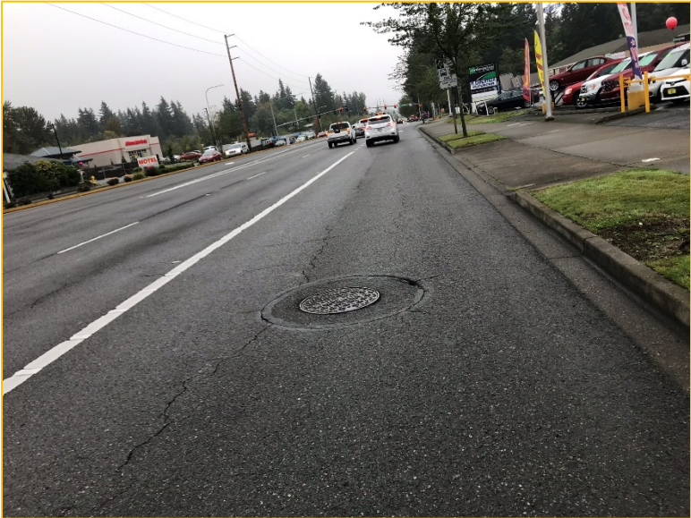
Photo 10A – Looking South – Runoff continues into the manhole located in Pacific Highway S at the approximate ¼-mile downstream drainage location.
