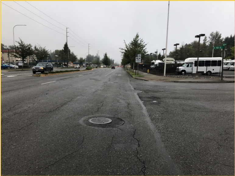
Photo 7A – Looking South – Flows enter the manhole from the east and are then conveyed south through a series of manholes in the southbound lanes of Pacific Highway South.
