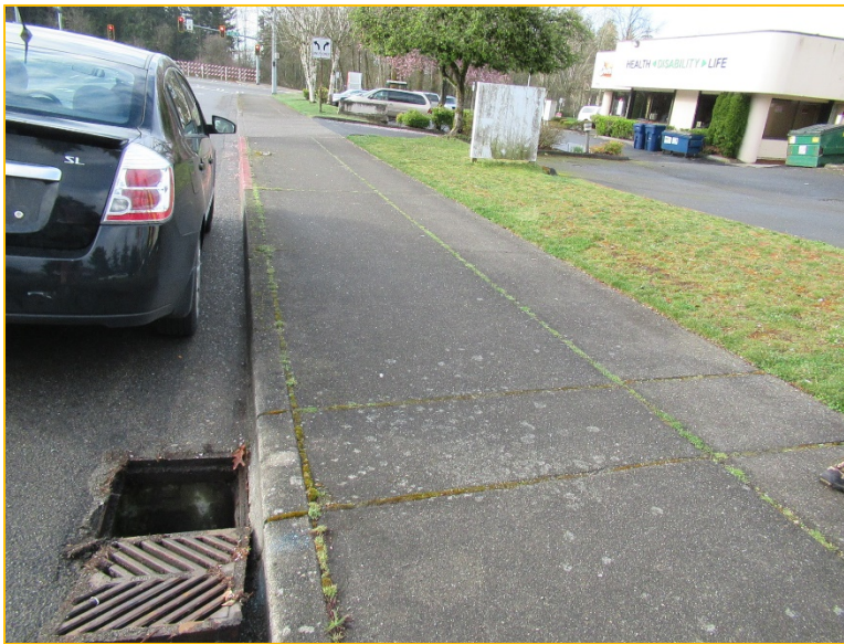
Photo 10B – Looking South – Flows continue south along the west side for 13 th Place South in a series of pipes and catch basins.
