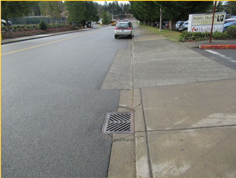
Photo 8B – Looking South – Flows continue south along the west side for 13 th Place South in a series of pipes and catch basins.
