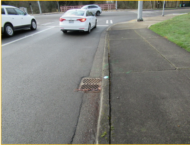
Photo 11B – Looking South – Flows continue south along the west side for 13 th Place South in a series of pipes and catch basins.
