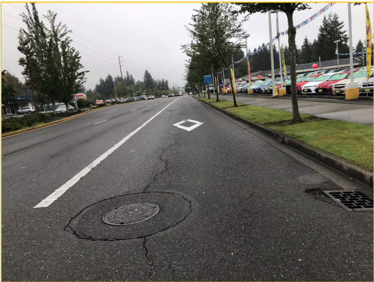
Photo 9A – Looking South – Runoff continues south through a series of manholes in the southbound lane of Pacific Highway South.
