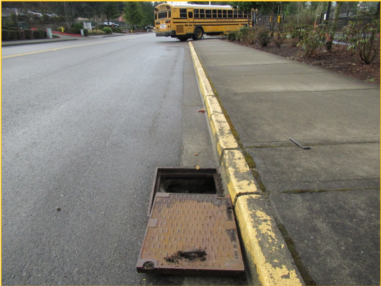
Photo 6B – Looking South – Flows continue south along the west side for 13 th Place South in a series of pipes and catch basins.
