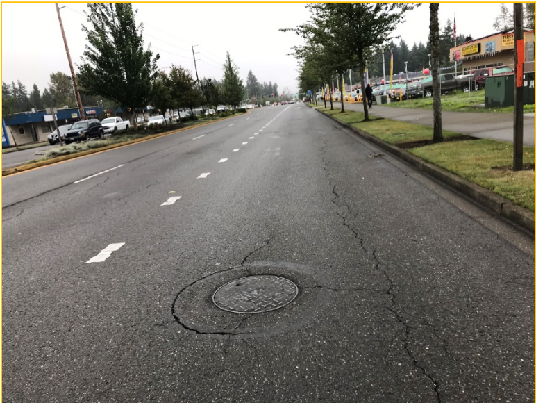
Photo 8A – Looking South – Runoff continues south through a series of manholes in the southbound lane of Pacific Highway South.
