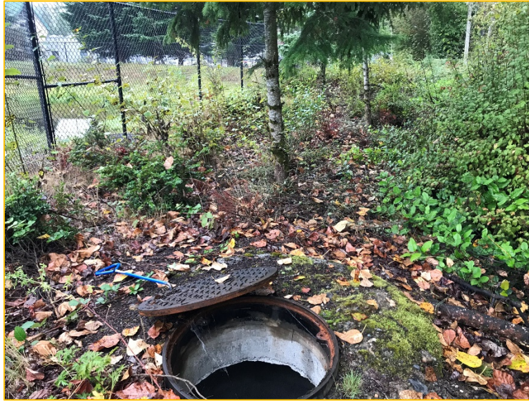
Photo 4C – Looking Southeast – Flows enter the stormwater manhole located on the northeast corner of parcel 9265010030 and is then conveyed southeast.
