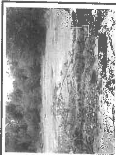
Photo #28 Offsite Parcel A Facing southeast Concrete slab of former auto wrecking yard, auto body shop, and an airplane hanger 6" diameter pipe in foreground
