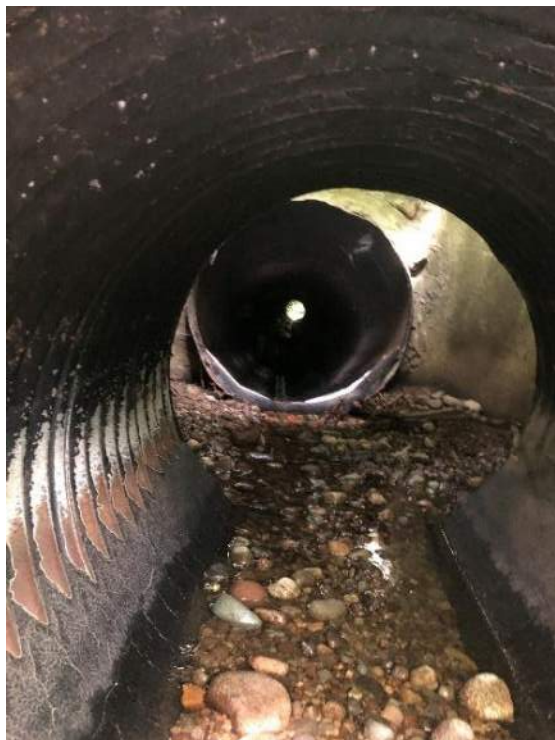
Photo 4 SR 509 View looking thru 36" CMP at inlet of 42" CMP.
