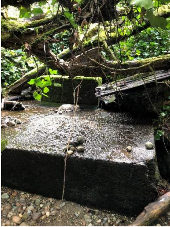
Photo 9 SR 509 perched outlet slab and flow dissipater wall.
