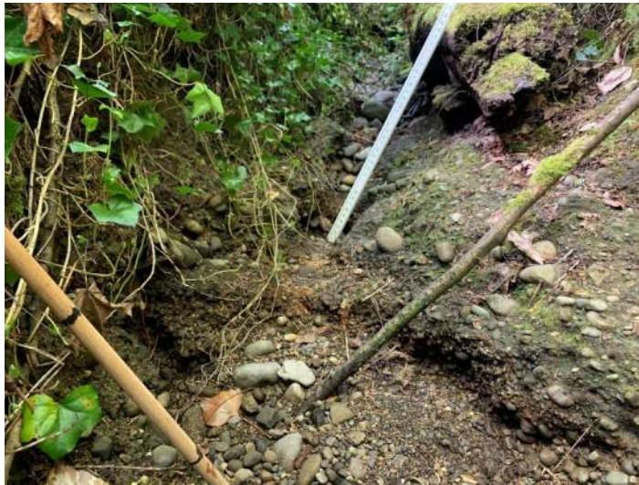
Photo 8: Looking upstream: scour and headcutting, exposing underlying geologic material.
