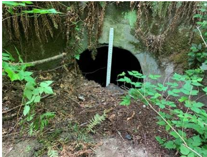
Photo 21: Unmapped culvert inlet, half blocked by debris, sand deposited upstream of inlet.
