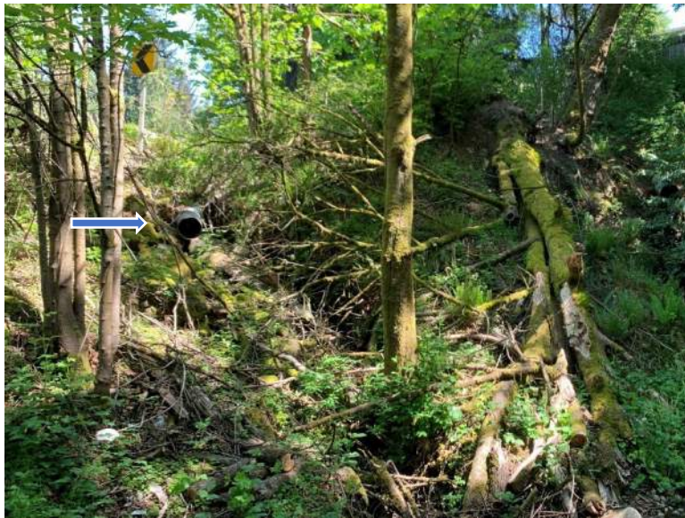
Photo 3: Stormwater input at Sta 6050; incised conveyance channel leads from outlet toward lower center of photo and then down to the left of the standing tree in the center of photo.
