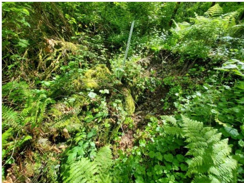
Photo 25: Separation of concrete pipe sections (marked with stadia rod) and erosion upstream of unmapped culvert outlet.
