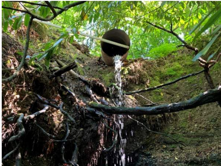
Photo 2: Stormwater pipe at Sta 6050 with 14-foot-high headcut bank
