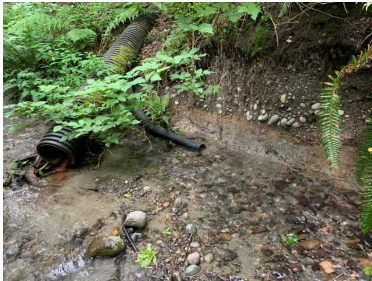
Photo 46: Local lateral scour.
