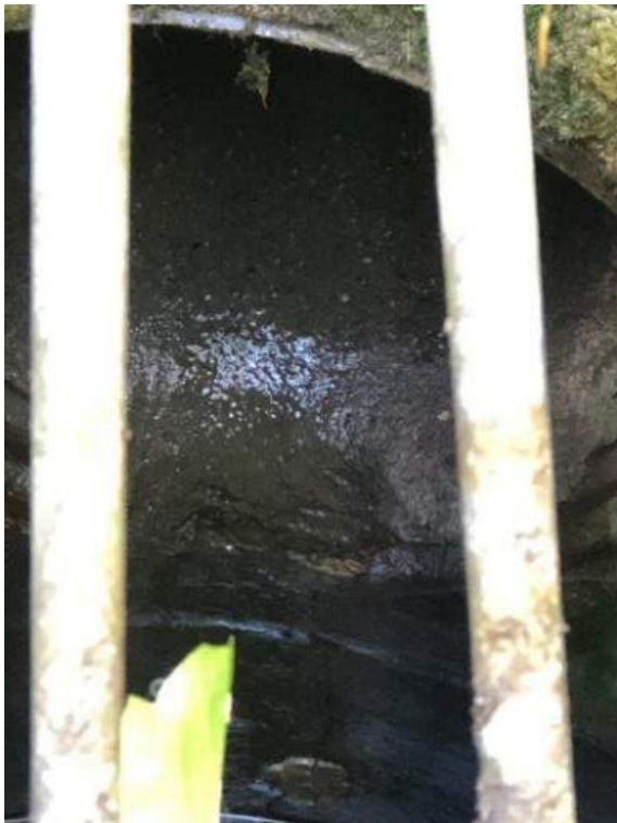
Photo 25 Outlet of Asset ID # 21522 between Asset ID # 21522 and ID # 21523. CMP Concrete Repair of Invert.
