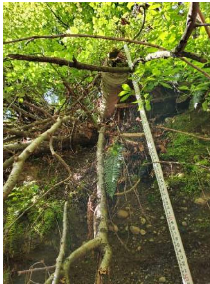
Photo 1: Stormwater input at Sta 6350 forming 12-foot-high headcut bank
