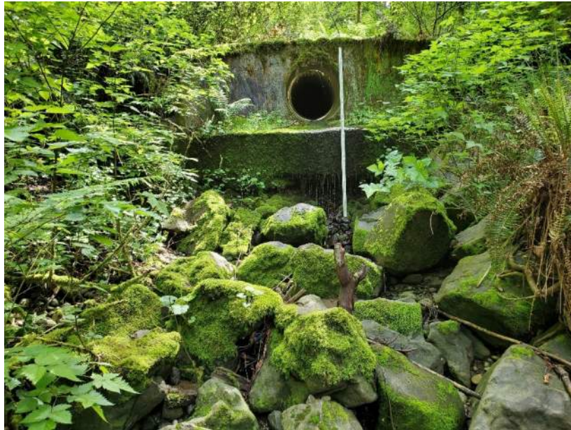
Photo 24: Outlet of unmapped culvert with boulder cascade. Apron is 2 feet thick. Refer to Photo 21 for view of inlet to this culvert.
