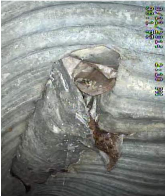
Photo 22 Asset # 21522 closeup of torn hole and debris.
