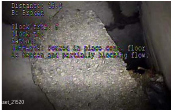
Photo 14 Asset ID # 21520 Broken bottom slab concrete stuck in bore.
