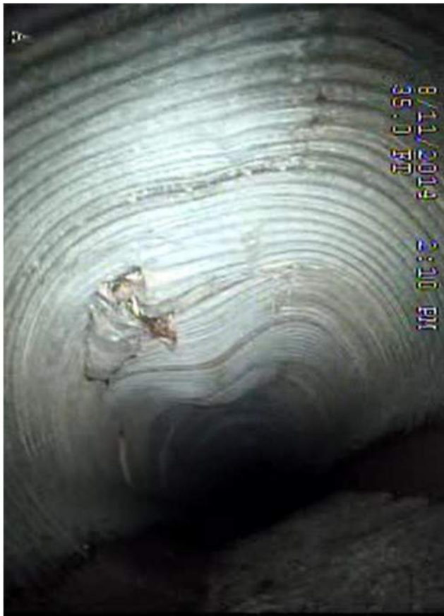
Photo 21 Asset # 21522 Crown damage at 35 feet. Hole torn in crown.
