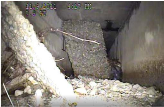
Photo 13 Asset ID # 21520 Broken bottom slab concrete stuck in bore looking upstream at 7.9 feet.
