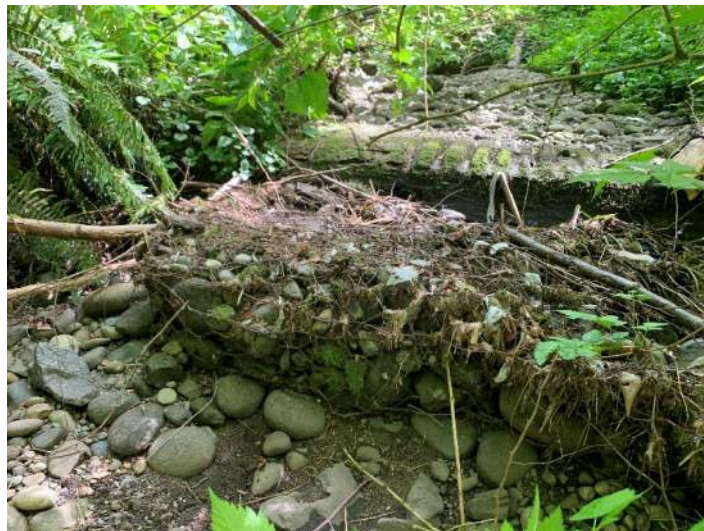
Photo 19: Notched log with wire gabion basket downstream.
