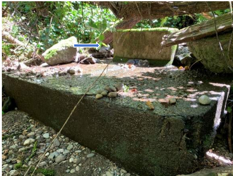
Photo 12: Concrete apron and flow dispersion structure (arrow). Apron has been flanked on both sides.
