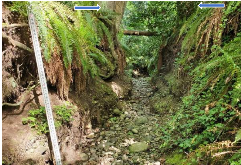
Photo 9: 6 feet of incision over time; approximately 2 feet of recent incision illustrated by vertical banks at edge of creek. Arrows indicate large trees that were once at the edge of and near the same elevation as the creek.
