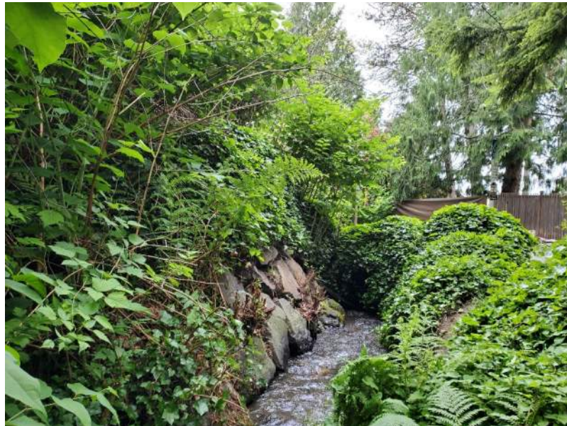
Photo 43. Culvert at downstream end of reach with rock armoring and invasive species.
