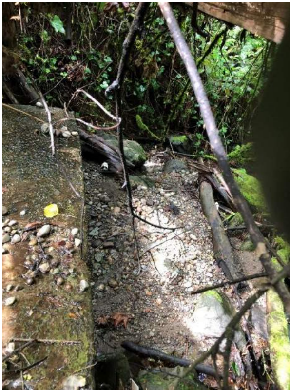
Photo 8 SR 509 Outlet slab perched end.
