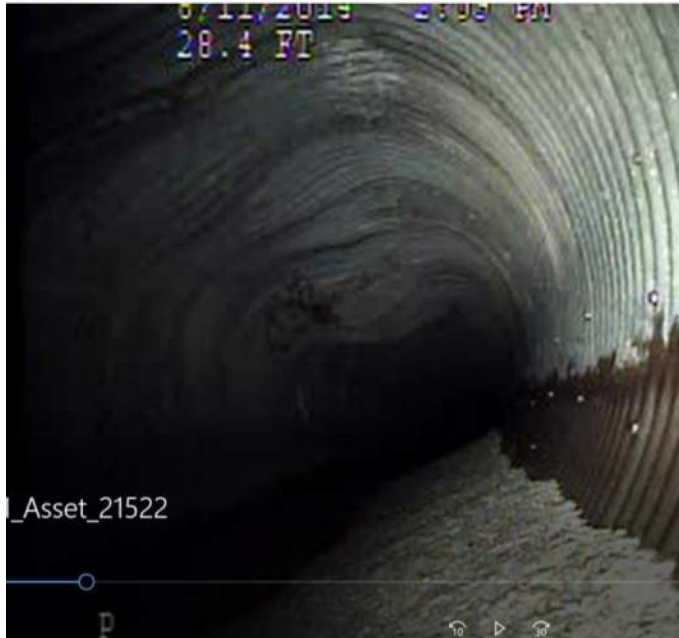
Photo 20 Asset ID # 21522 crushed CMP crown at ~22 feet.
