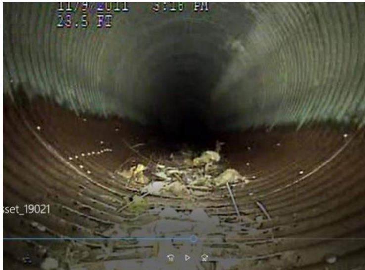
Photo 15 Typical heavy corrosion in CMP invert. Note the holes in the invert.
