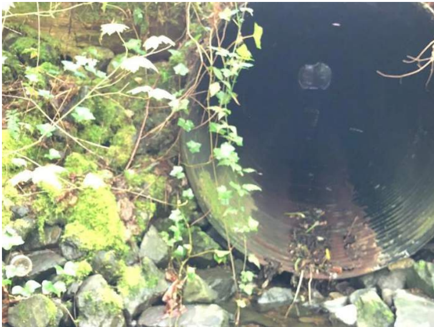
Photo 27 Outlet Asset ID 21523 corrosion at invert.
