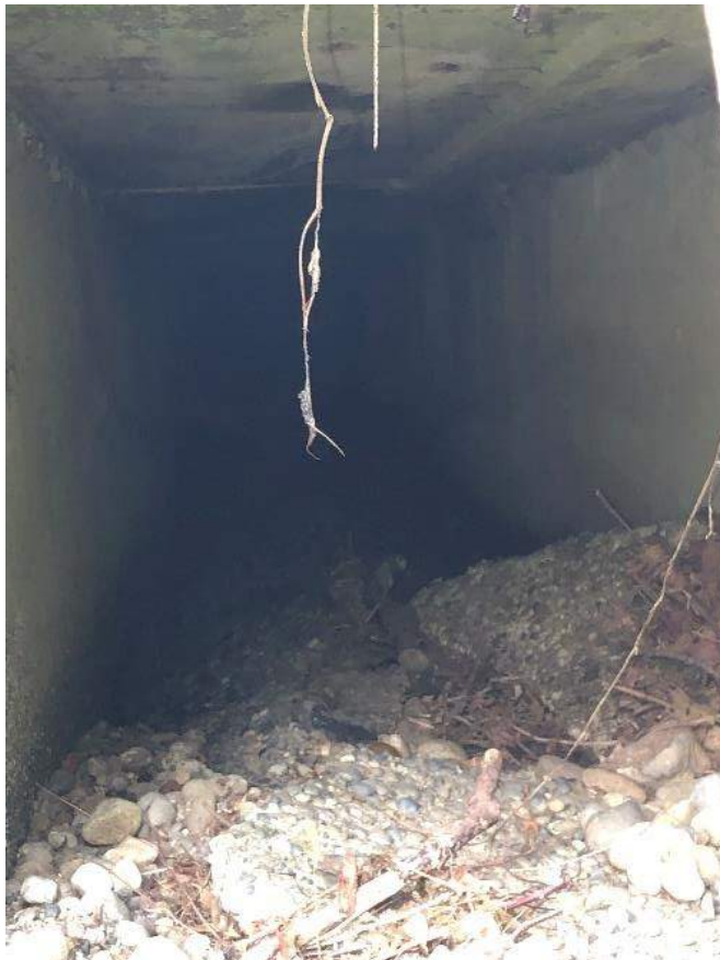
Photo 12 Marine Hills ID # 19017 Inlet Bore bottom slab broken pieces.
