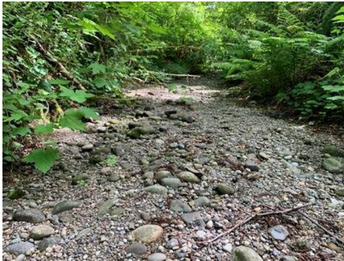
Photo 22: Sediment filled channel downstream of grade control but upstream of unmapped culvert.
