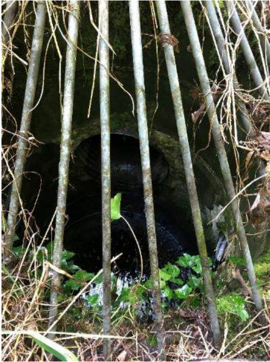
Photo 24 Asset ID # 21522 outlet CMP at manhole between Asset ID # 21522 and ID # 21523.
