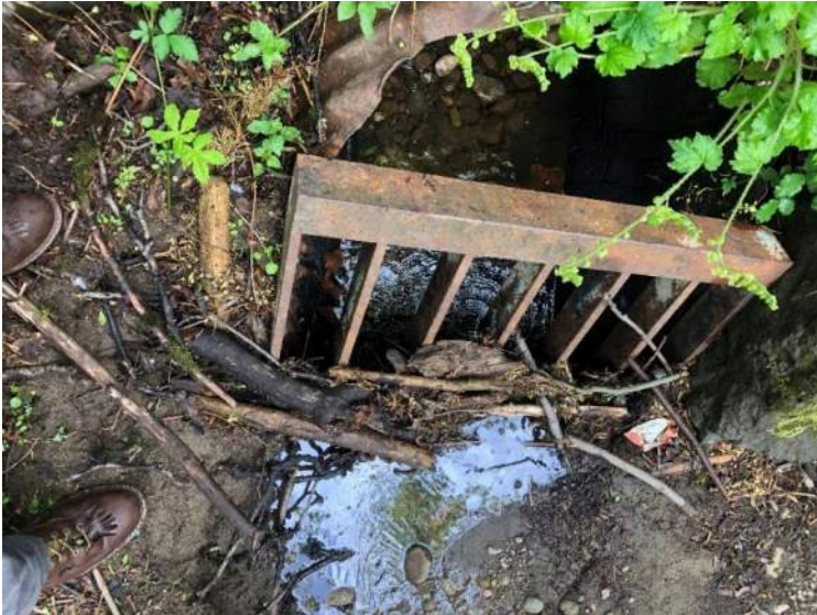
Photo 1 SR 509 36" CMP inlet and steel grate. Stream bed is filled in ~18 inches above CMP invert.
