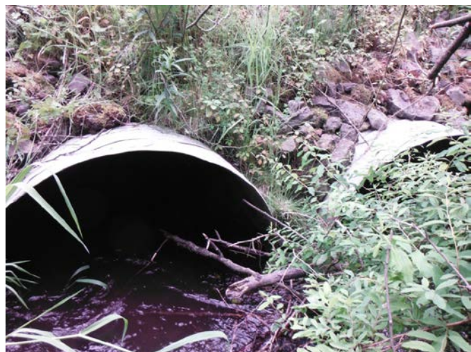
Figure 7: Culvert under 356th St in need of replacement, West Hylebos (HDR Engineering)
